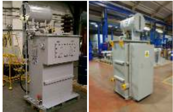
Gantry (Structure) Mounted
